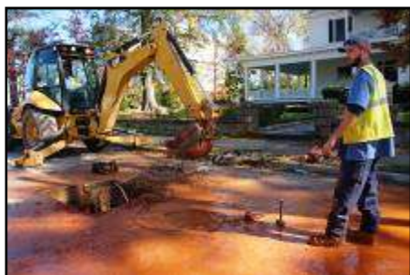
Roy Gardner stands in wet, red clay mud as work continues on a leak under Macon Street.
