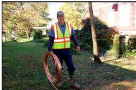
Ron Harris feeds line under the road as needed to get this job done.
